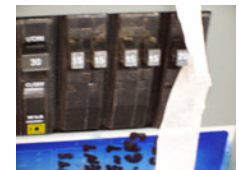
Breaker box for all interior lighting
